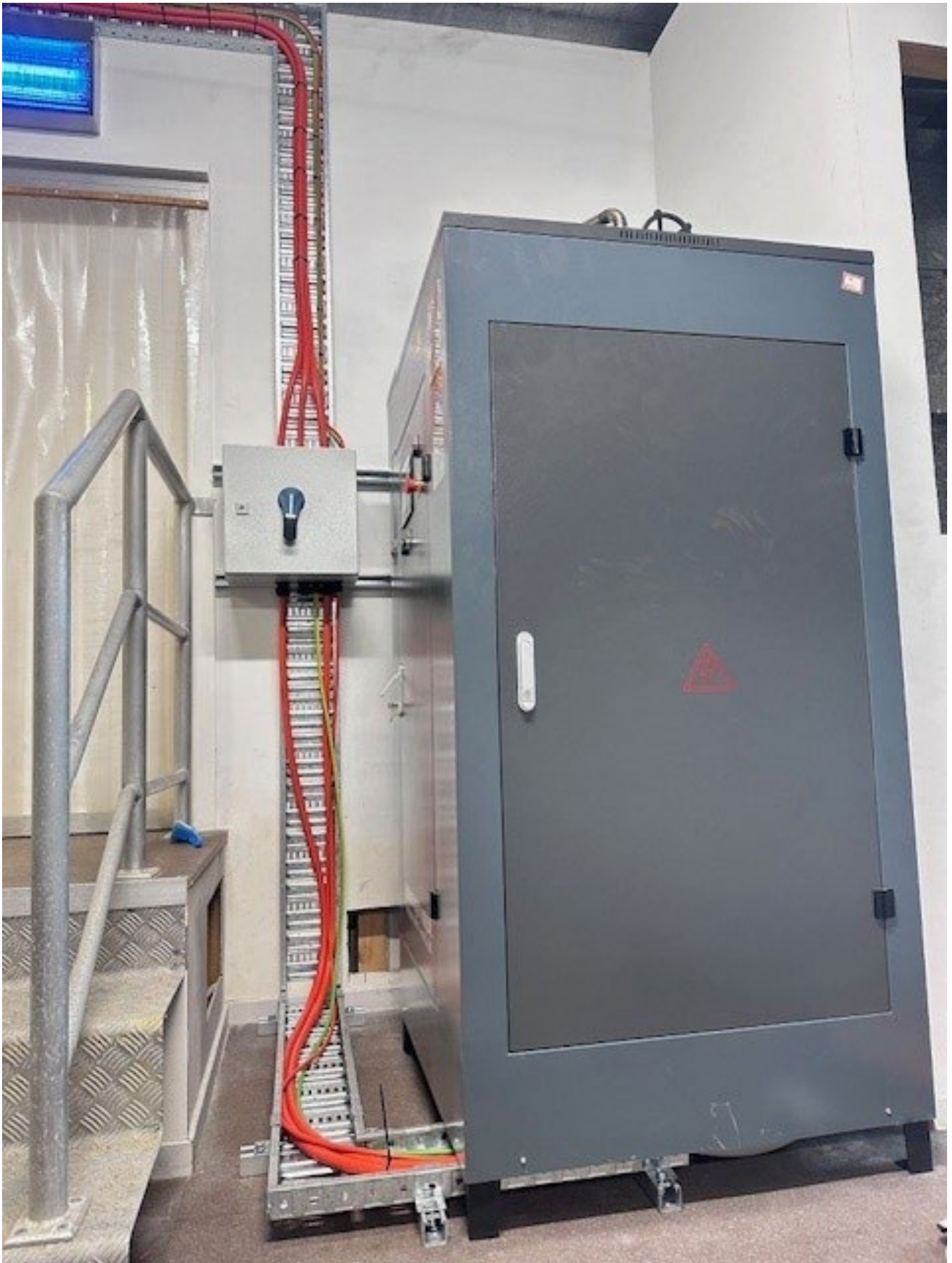
Figure 2: Steam generator. Source: Tas Live Abalone Pty Ltd
